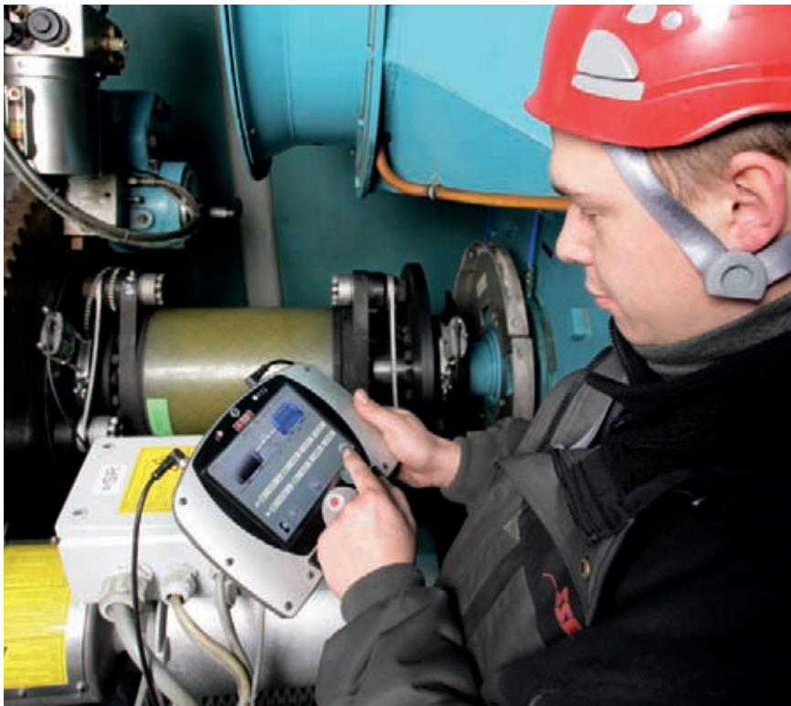
SSB service technician aligning an insulated coupling.
